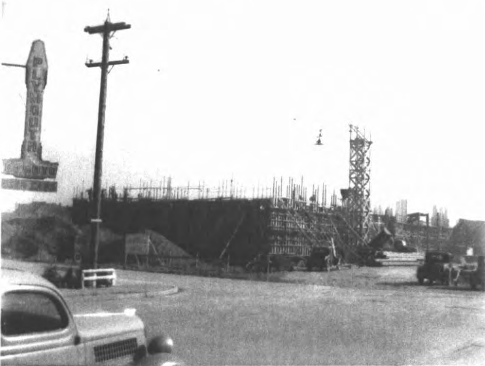
Bellingham City Hall, preliminary construction, circa 1939 Photo courtesy of the Whatcom Museum of History and Art in Bellingham, Washington.
